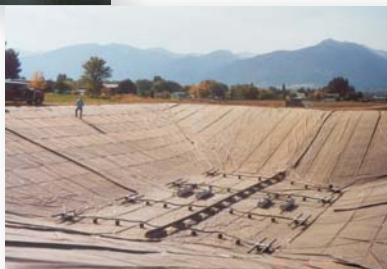
Sub-Surface Aeration Diffusers
